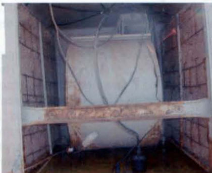
Fig. 3. The effect of the cumulated salt on the evaporative cooler (inside the cooler).
