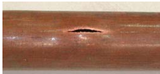
Fig. 14b: The rupture on the hard temper 1.25" (31.8 mm) copper pipe.
