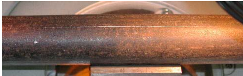
Fig. 17a: The line of fracture on the seam of the MS pipe of OD=26.67 mm, t=2.87 mm.
