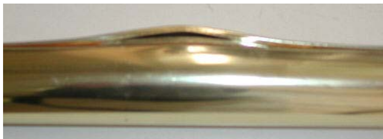
Fig. 13a: The splitting of the seam in the aluminum pipe.
